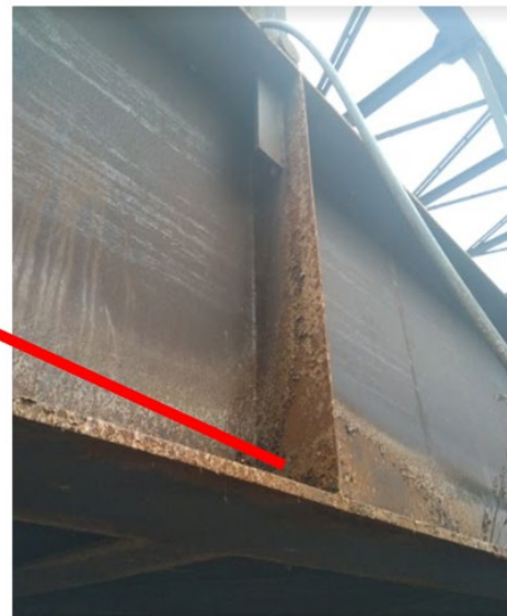
Figure 6. Oxidation and corrosion evidence found on the web stiffener of the main girder element of the Unete steel arch bridge
