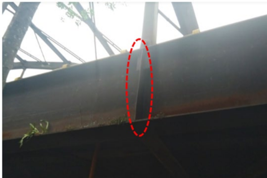
Figure 7. Local buckling of a web stiffener just at the point of a hanger’s connection area for the Unete steel arch bridge
