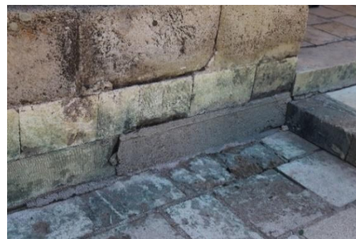
Figure 9. A sample for Insulation/humidity problems of exterior walls.
