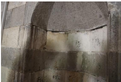
Figure 6. A sample of broken/spilled stones in the interior wall.
