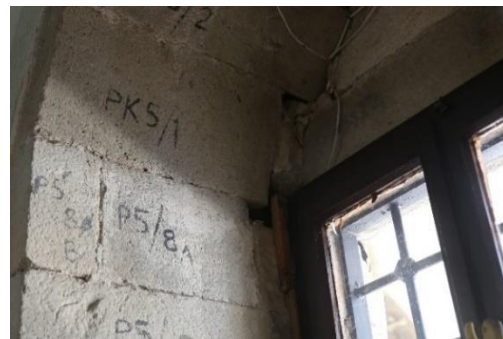
Figure 7. One of implementation defects at the stone joints in the interior.
