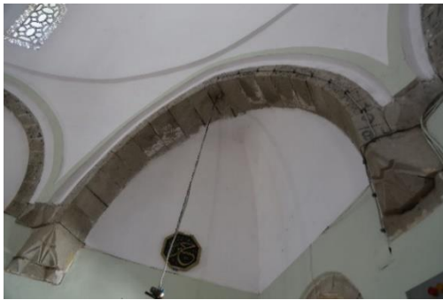
Figure 4. Deficiencies in the joint filling of the arch elements in the interior.
