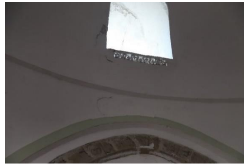
Figure 5. Humidity/insulation problem of the windows in the dome.
