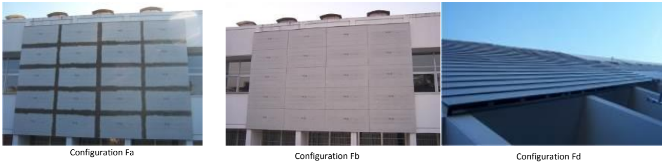
Figure 7. Diagram of the opening degree adjustment for ventilation. The intermediate air chamber ventilates through the upper and lower edges of the tested LVF façade section. The opening levels of the surface used to ventilate the intermediate air chamber are: 1 = 0% opening surface, 2 = 25% opening surface, 3 = 50% opening surface, 4 = 75% opening surface, 5 = 100% opening surface. A is the assembly of the LVF system, B is the lightweight system and C is the base wall. (Source: compiled by authors).
